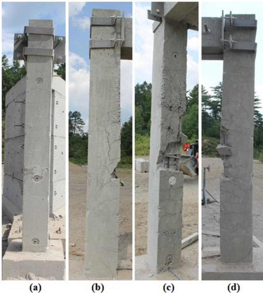
Figure 4-25: Post-test photograph of Column SEIS-9 faces: (a) Front face, (b) Side face (right) (c) Back face, and (d) Side face (left)
