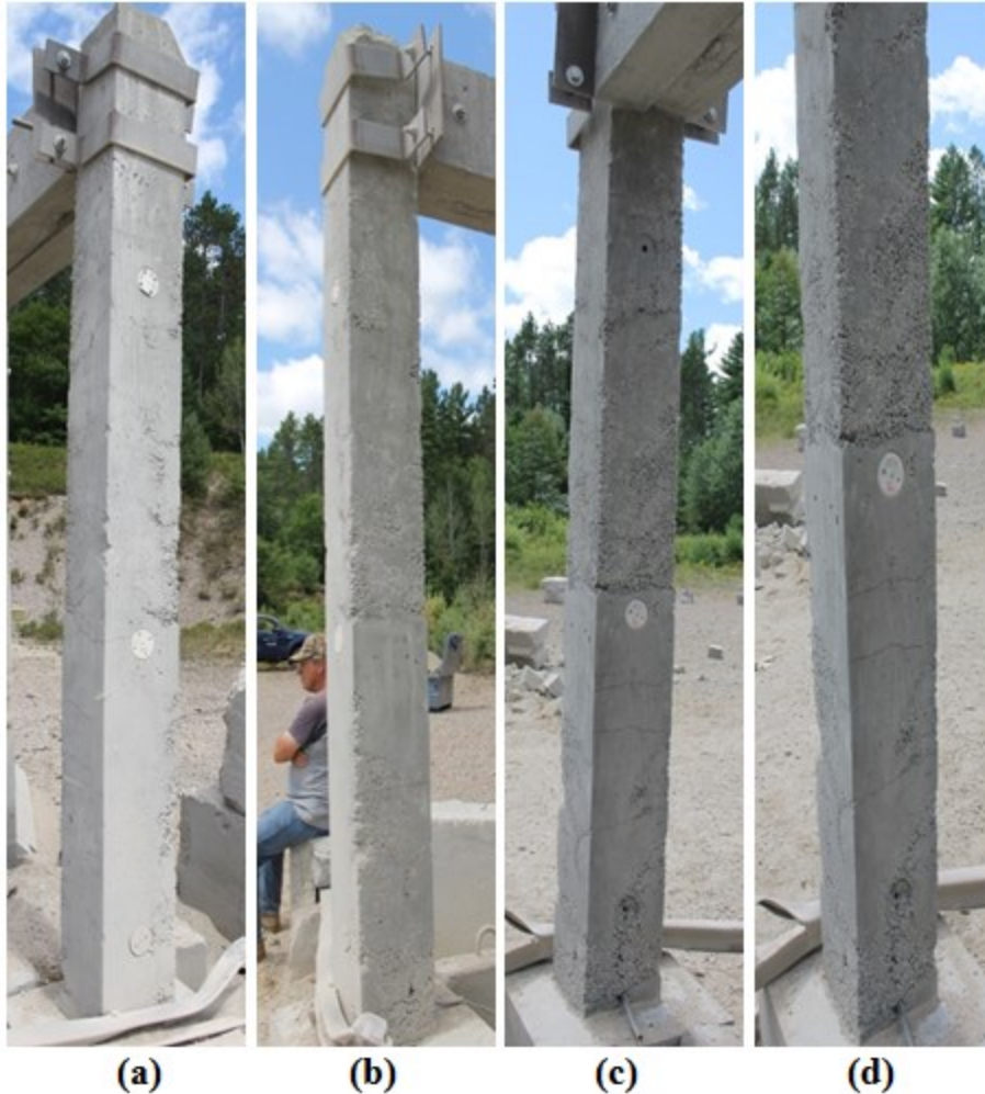
Figure 4-64: Post-test photograph of Column CONV-12 faces: (a) Front face, (b) Side face (right), and (c, d) Back face
