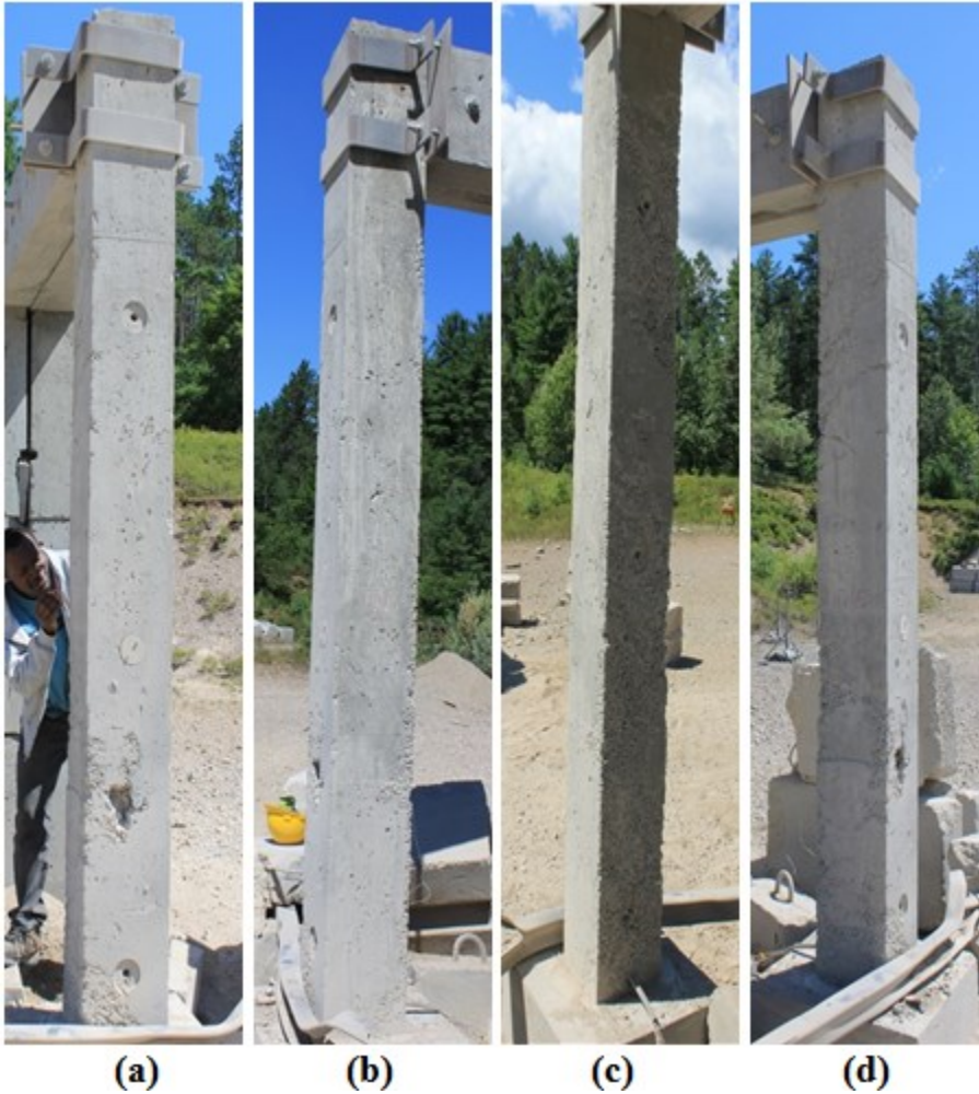
Figure 4-69: Post-test photograph of Column CONV-15 faces: (a) Front face, (b) Side face (left), (c) Back face, and (d) Side face (right)
