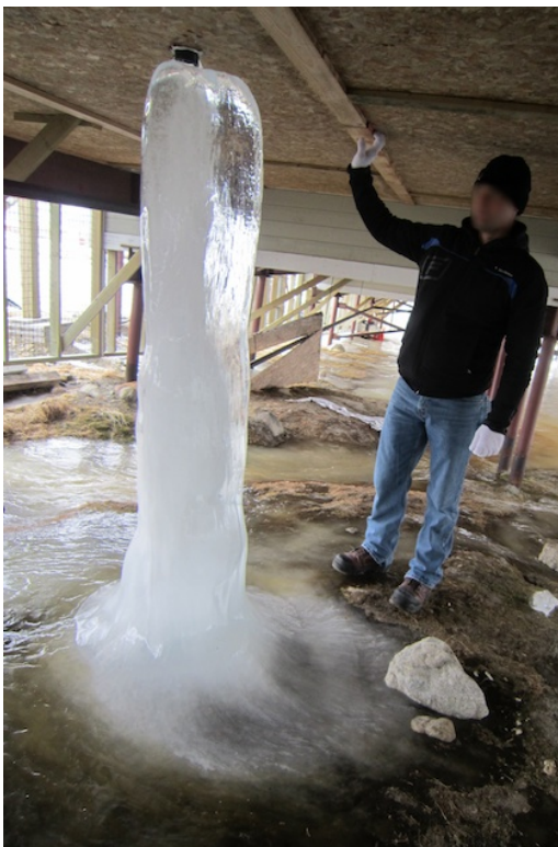
Figure 5.21 – Clogged drainpipe under building
