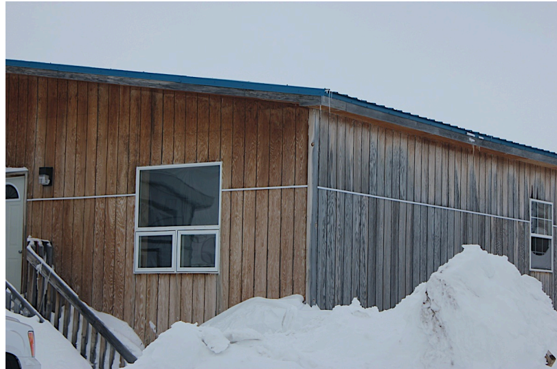
Figure 4.10 – Solar damage on south facing wall
