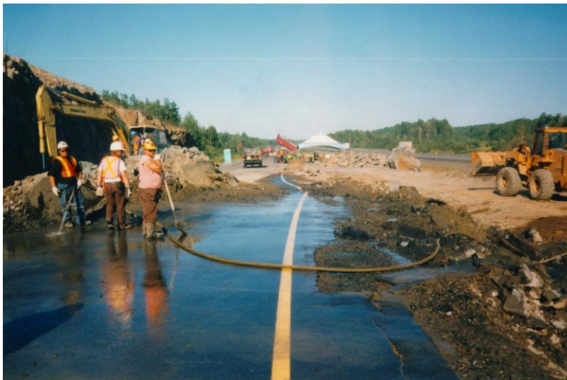
Figure 119: Highway asphalt shifts as a result of the huge explosion (Provencher, 2005)
