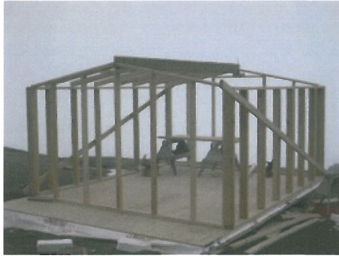
Figure 4.4 Construction of a new cabin at spring camp, Nasauyak Point (Spring Camp, May 2010, Gita Ljubicic)
